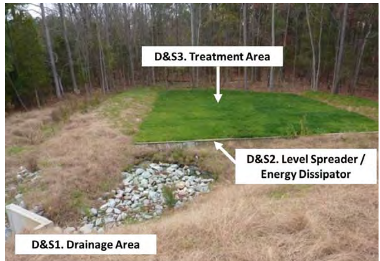
Figure 2.4.1 Key Areas for Level 1 Inspection of Disconnection and Sheetflow with filter strip shown.
