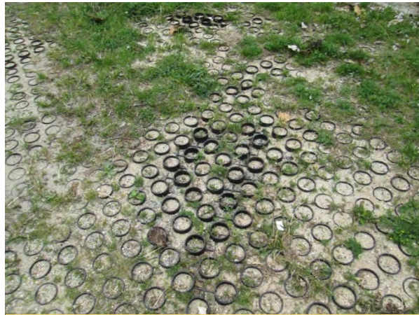
Figure 3.9.2. A Level 3 investigation is warranted if more than 25% of the permeable pavement surface appears to be clogged, or joints are filled in, or, as shown in the photo, vegetation is growing.
