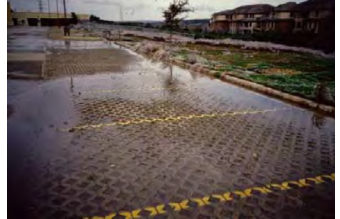
Water standing on the parking surface 48 to 72 hours after a storm is an indication of clogging. Snow piles at the edge of the photo point to possible clogging from winter sanding or plowing.
