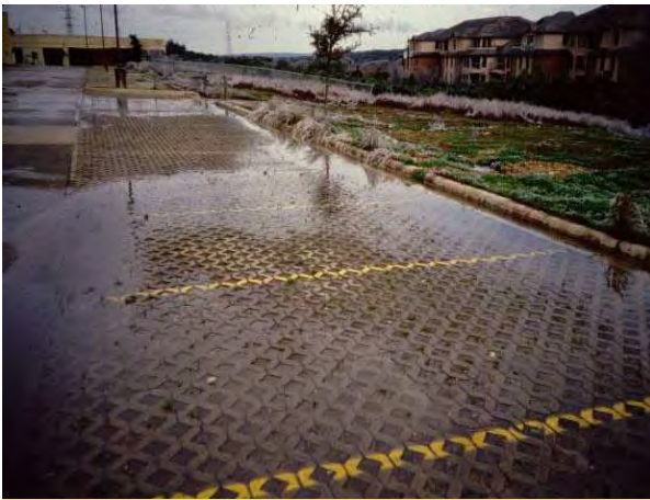
Figure 3.9.1. Winter salting, sanding, plowing, and snow storage can cause problems for permeable pavement surfaces, which will trigger a Level 3 investigation.
