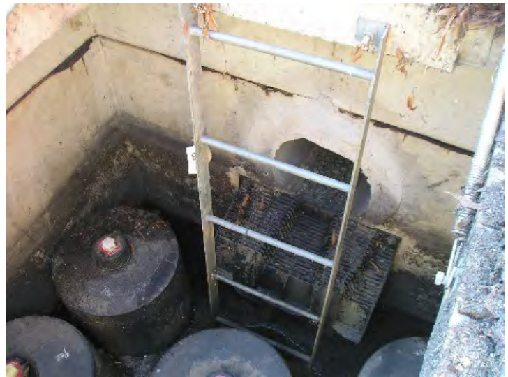
Figure 2.12.2. Examples of underground filters: Left –Perimeter sand filter in a concrete box (photo shows the filter with the grate top off as the filter is being maintained). The right-hand side is a sedimentation chamber filled with water and the left-hand side is the sand filter chamber. Right –Underground vault filter with special organic filter media inside cartridges.
