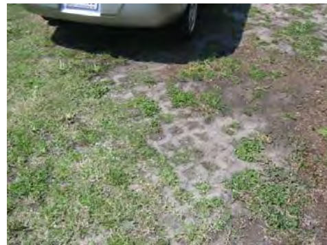
Pulling grass and weeds from the joints can damage parking surface if roots are firmly established in the bedding layer.
